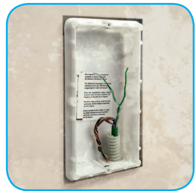
Use of an existing pair of wires to connect the new entrance panel
