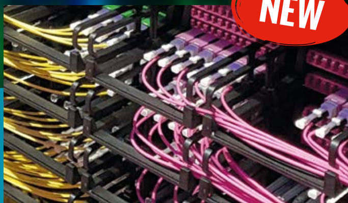
HIGH-DENSITY DATA CENTRE SOLUTION (HD-DCS)
